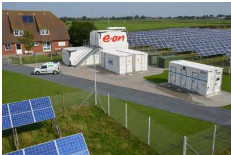
Figure 4: Distributed electrical storages at Pellworm
