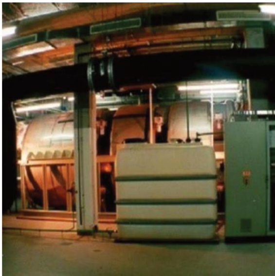
Figure 2: Zeolite sorption storage in the district heating network of Munich, Germany (© ZAE Bayern)
