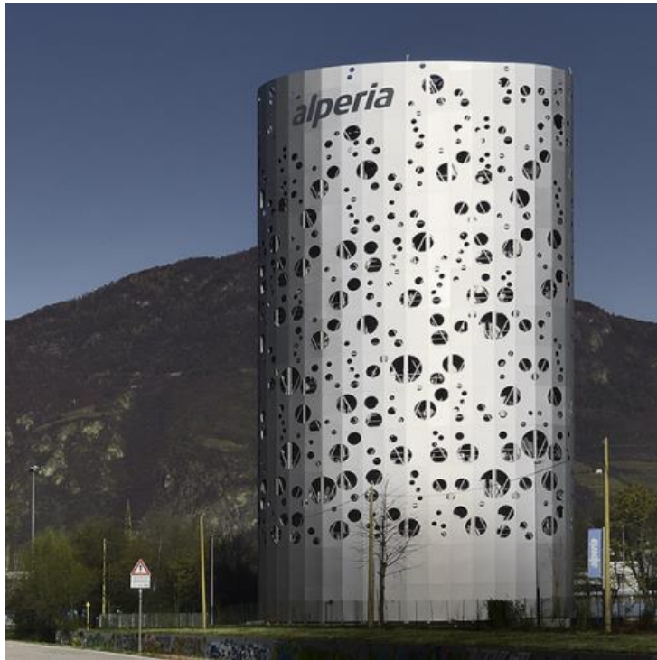
Figure 2: 5,600 m 3 hot water storage tank in Bolzano, Italy (© Alperia SpA)
