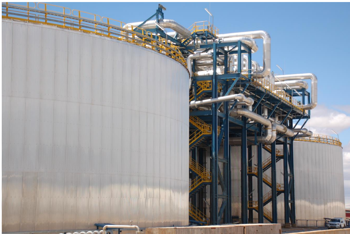
Figure 2: Liquid salt storage in a solar thermal power plant (source: Andasol 3)
