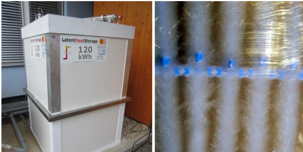
Figure 4: Latent heat storage for recooling of an absorption chiller used in solar air conditioning (l.), PCM crystallising on heat exchanger during discharge of storage (r.) (© ZAE Bayern)
