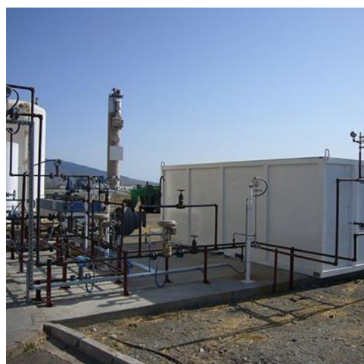
Figure 3: 100 kW latent heat storage module, charging with solar-generated steam. Binary nitrate salt mixture as storage material, phase change at 220 °C.
