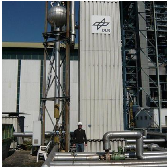
Figure 1: Latent heat storage module with 700 kW power, storage capacity 1 h, \text{NaNO}_3 as storage material, phase change at 305 °C
