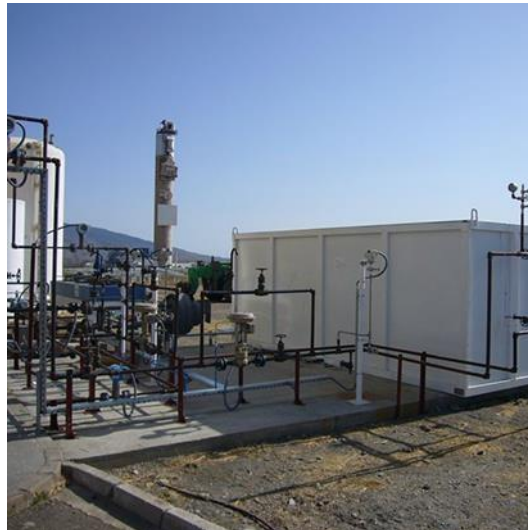
Figure 3: 100 kW latent heat storage module, charging with solar-generated steam. Binary nitrate salt mixture as storage material, phase change at 220 °C (© DLR)
