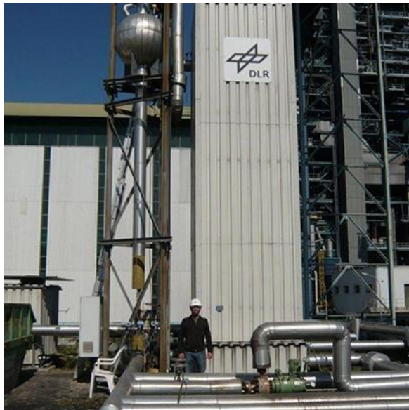
Figure 1: Latent heat storage module with 700 kW power, storage capacity 1 h, \text{NaNO}_3 as storage material, phase change at 305 °C (© DLR)
