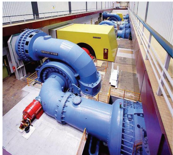
Figure 2: Ternary machine set at Kraftwerk Wehr, Germany (© Schluchseewerk AG)
