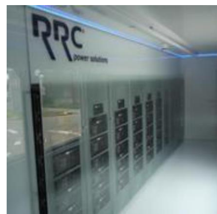
Figure 3: Electricity storage container by RRC power solutions for buffer storage and emergency power supply at a municipal site in Saarland, Germany (© RRC power solutions GmbH)
