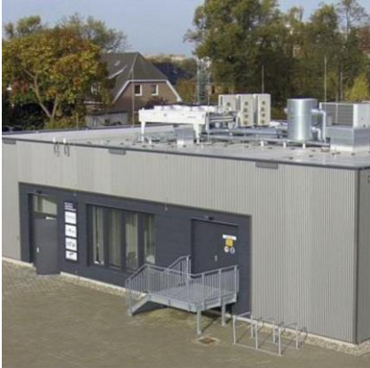
Figure 4: WEMAG storage, 5 MW/5 MWh, participating in the primary control energy market, first commercial battery storage in Europe, situated in Schwerin, Germany (© Younicos AG)
