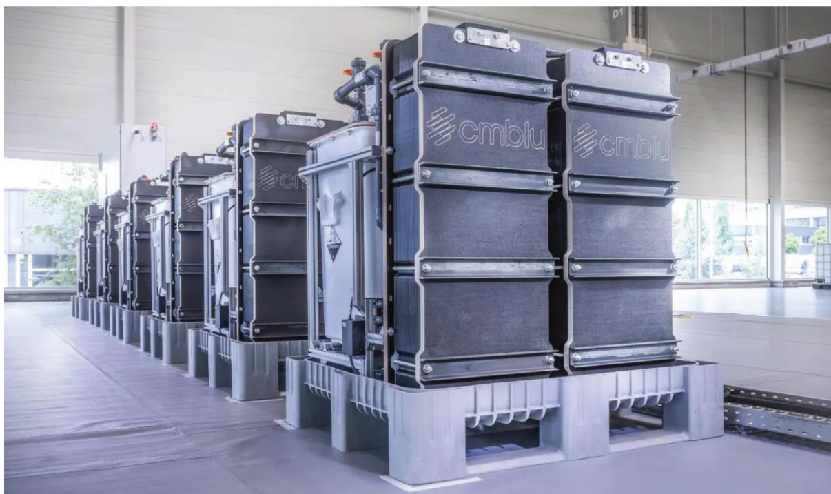
Figure 1: Organic-flow battery arrays with dark grey stacks in front and electrolyte tanks in the back (© CMBlu)
