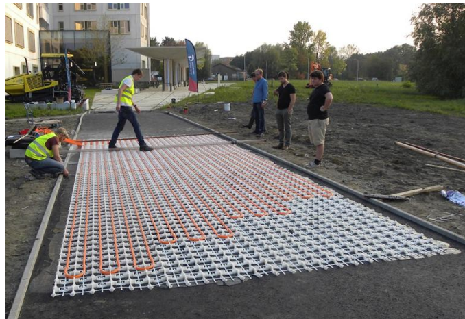
Figure 4. Pipe and grid placement in HEAL project at the University of Antwerp
