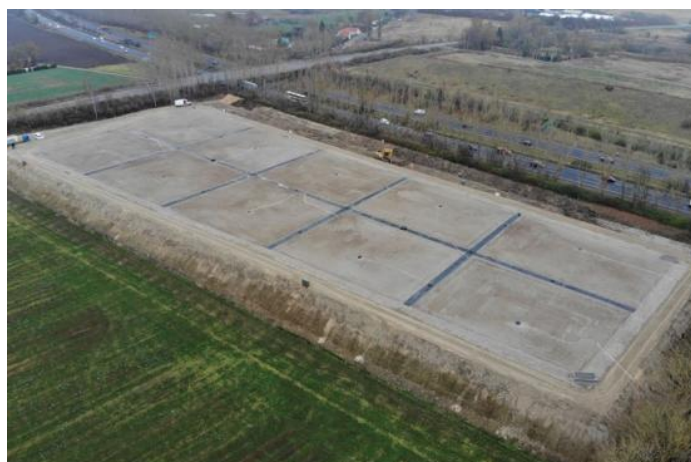
Figure 5-4: Pit thermal energy storage in the Høje Taastrup Project, Denmark (Photo: Ioannis Sifnaios).
