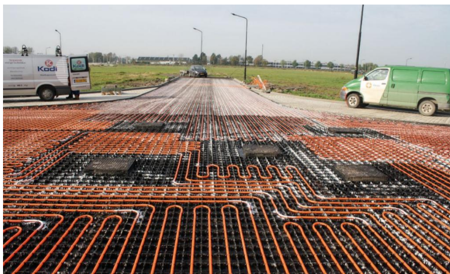
Figure 8. The construction stage of HHP with grid support in a RES project ( Lieshout 2017 )
