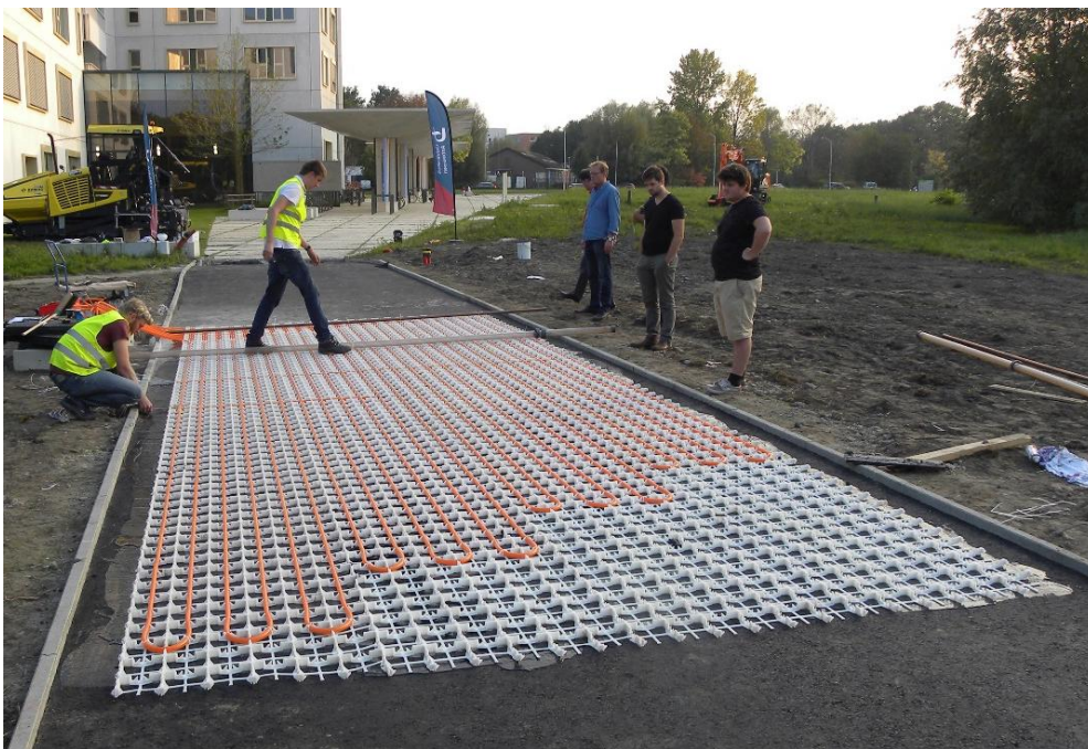
Figure 6. Pipe and grid placement in HEAL project at the University of Antwerp
