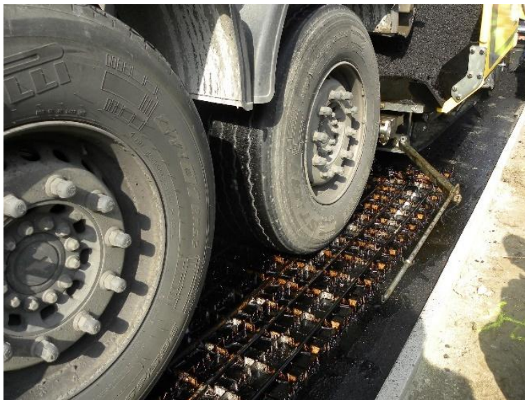
Figure 23. The pipe and grid structure in HEAL prototype at University of Antwerp, Belgium during asphalt placement
