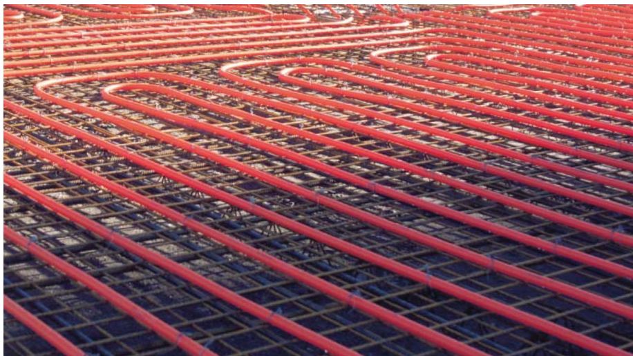
Figure 2. HHP pipes fixed to a mesh of rebar and ready to be cast into concrete (Uponor)
