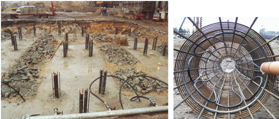
Figure 2. Pile top and fitted outlets of an energy pile (on the left), circulation pipes inside of the reinforcing cage (on the right)
