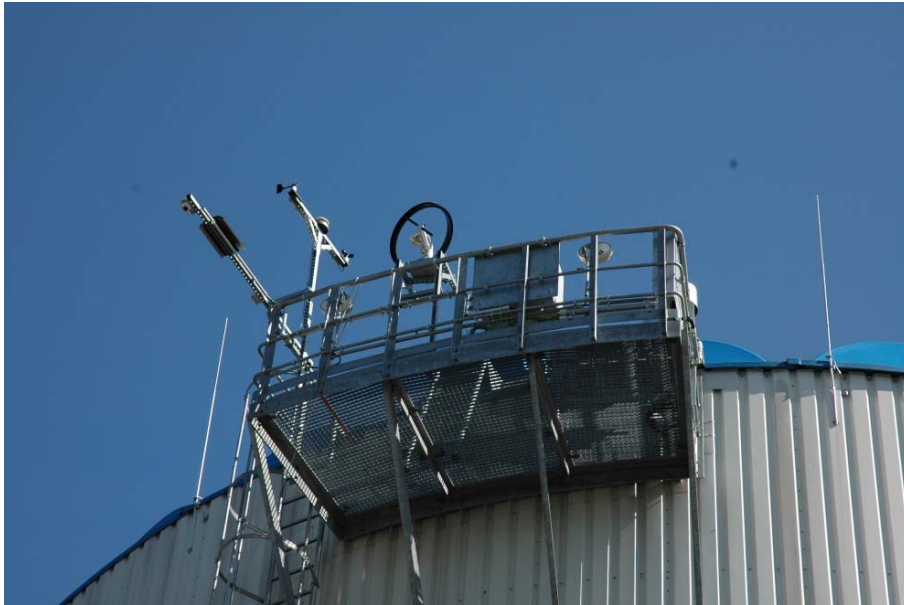
Figure 8: Weather station on top of cold water TES
