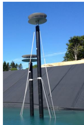
PTES diffusers in Dronninglund. Picture: PlanEnergi
